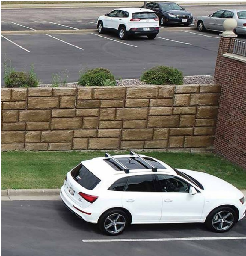
Bronco 30H Wall Units Stained
